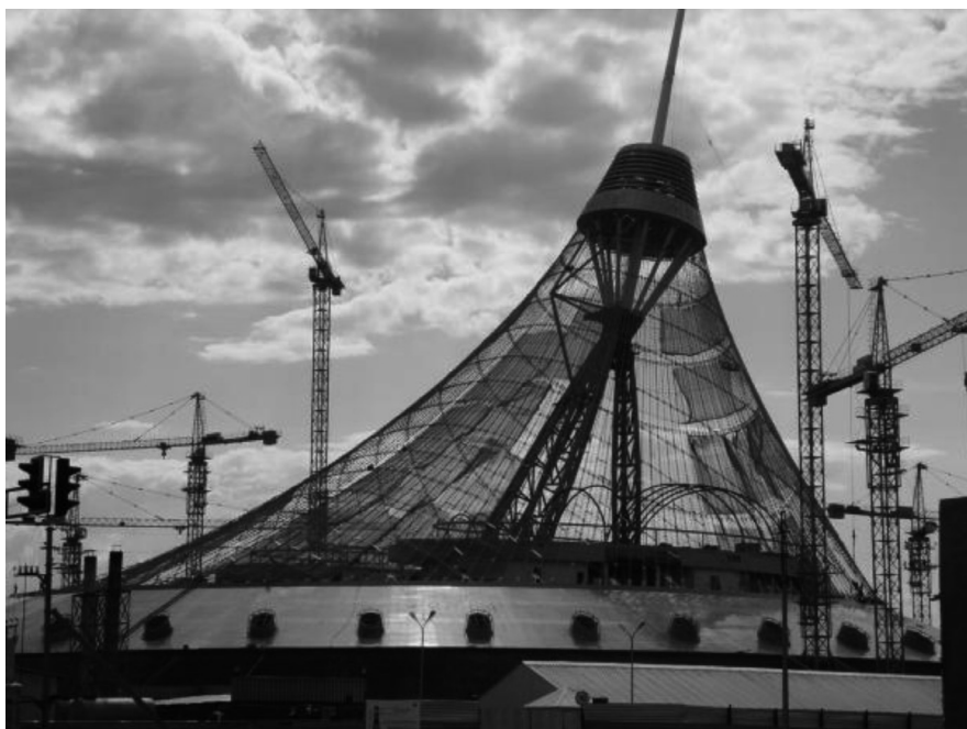
III. 3. A general view of the “Khan Shatyr” during the construction period (source: Conceptual design of Khan Shatyr, Foster and Partners)
