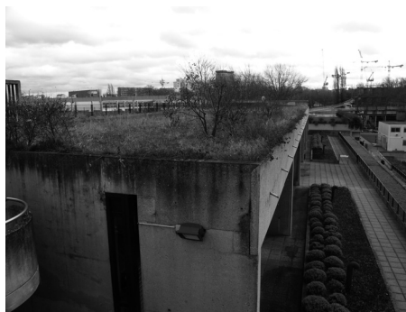
III. 7. The damages of parapet walls of flat roofs (photo by B. Siedlecki)
