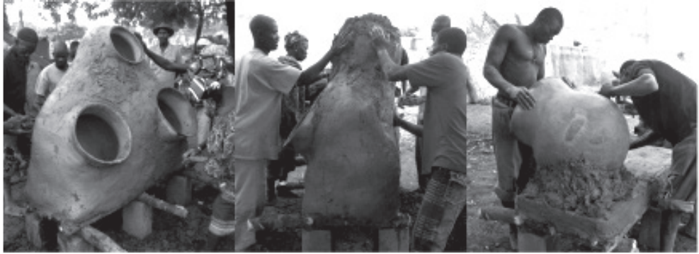
Ill. 18. Women's Association Centre in Gando. Burkina Faso. Casting of clay vessels used to store food products in the wall (source: [7])
