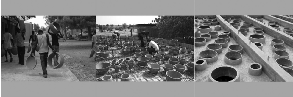
Ill. 16. Library in Gando. Burkina Faso. From left: Arranging trimmed ceramic vessels in the reinforcement of the floor slab and the finished floor (source: [2])
